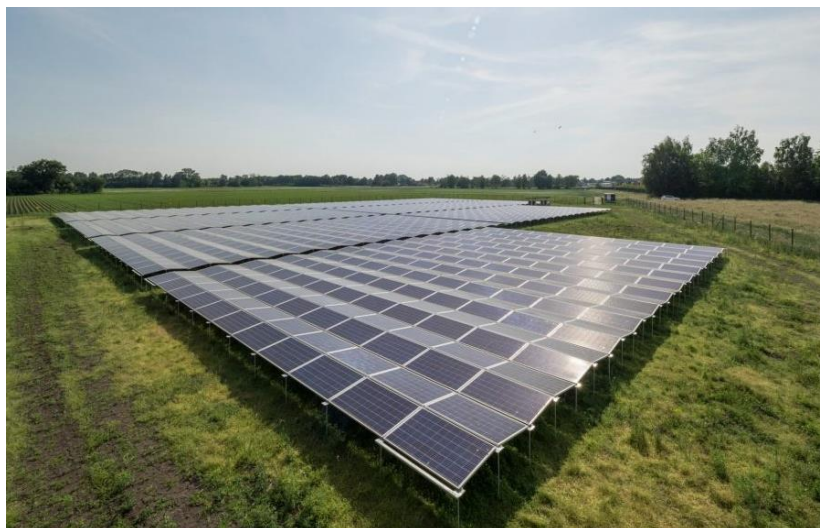
Figure 1. The PEG mounting structure comprises rows of alternate facing modules (photo courtesy of Belectric, n.d.)
